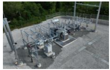
Substation at the Jeannette plant
