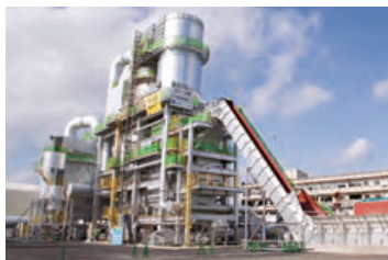
Temporary Incinerator in the Miyagi Kesenuma Block (Hashikami District)
