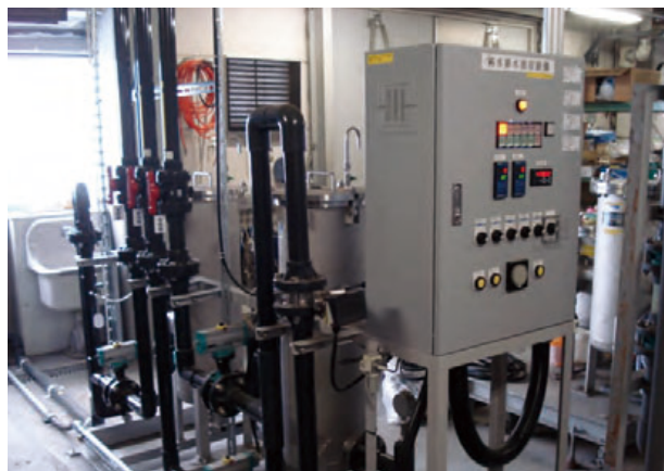
Deionized Water Recycling Equipment
